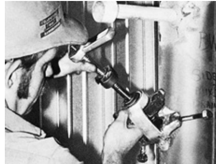
New stem/disc assembly is lowered into valve body after completion of reseating cuts.
