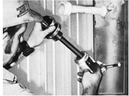
Reseating tool is lowered into valve body after removal of yoke bushing and valve stem.
